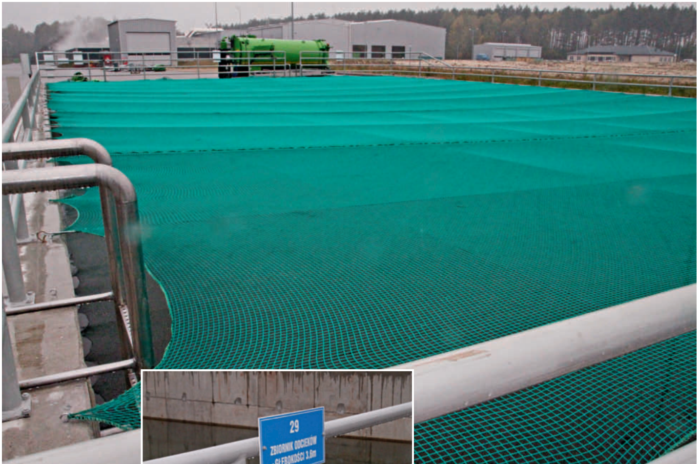
Process water store ▲ Prozesswasserspeicher
